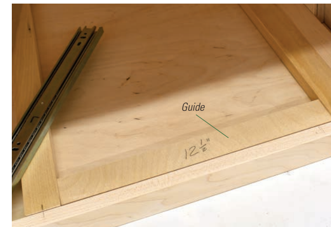
There's no better way to ensure that spacers for the drawer and shelf slides are aligned than to use guide pieces cut to the desired measurements. Install one side, then use the same guides for the opposite side.
